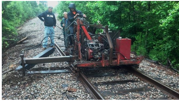
The track crew performs track work with the aid of the tie handler.
